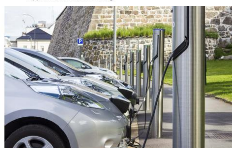
Electric vehicle charging points
